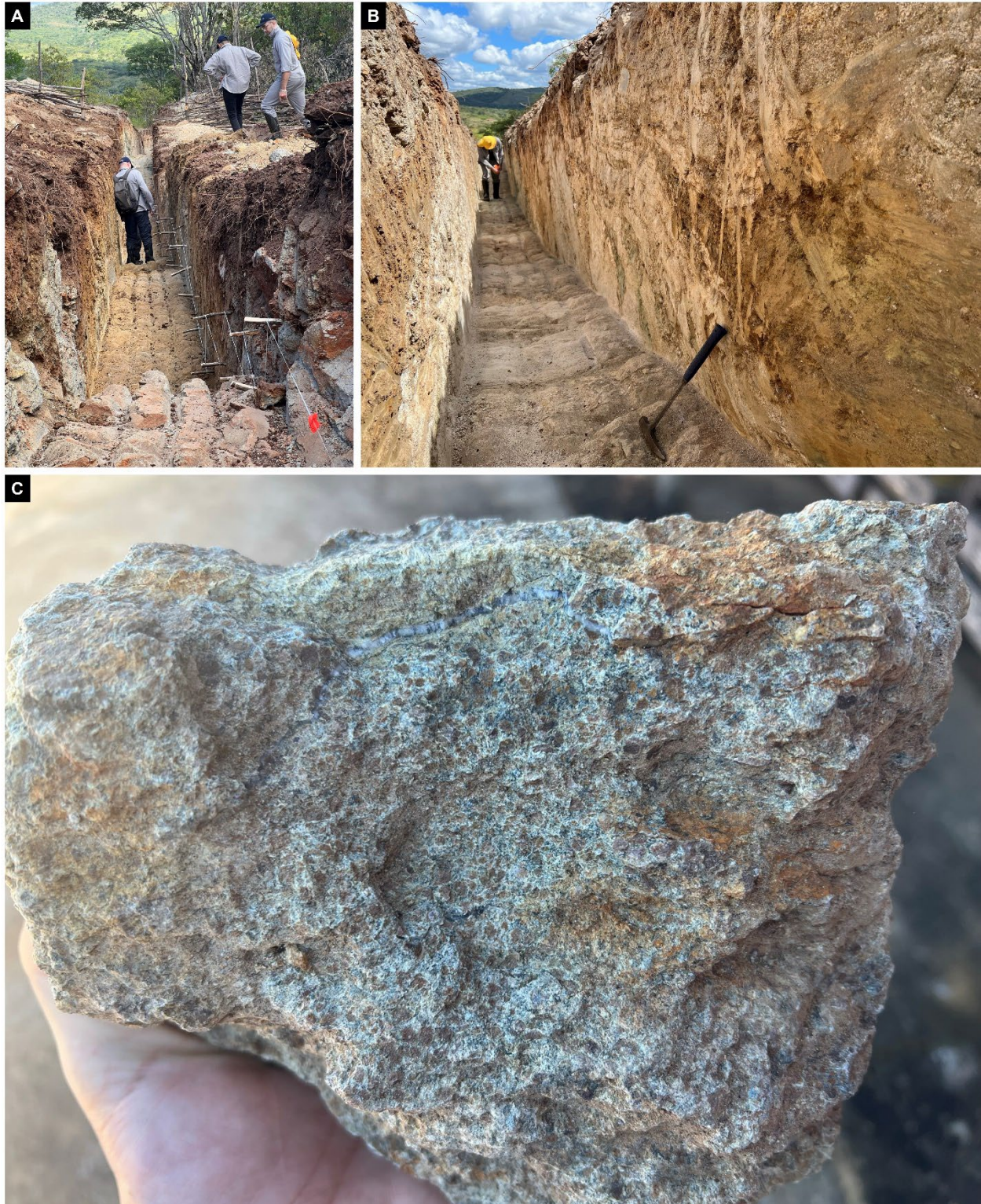
Figure 2: Photographs from trenching at Galante East (A and B), and a chromite-rich peridotite sample (C) collected at trench TR22GE01 from an interval assaying 1.07 g/t 2PGE+Au over 6 m.
